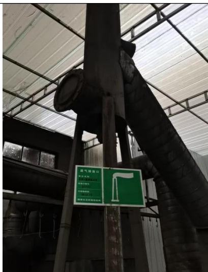
排气筒 DA001 (喷塑、抛丸)
